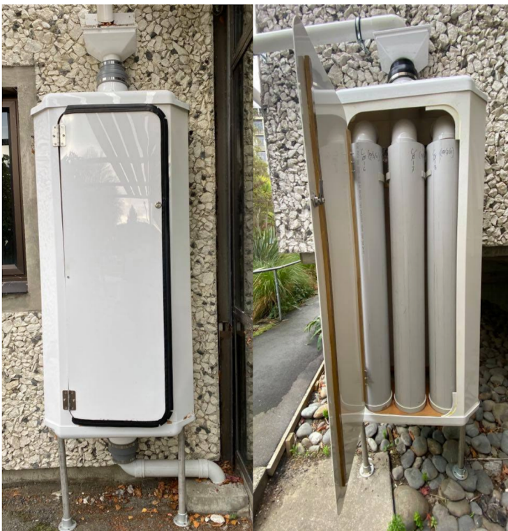
Storminator treatment system cabinet, and Storminator internal filter cartridges
